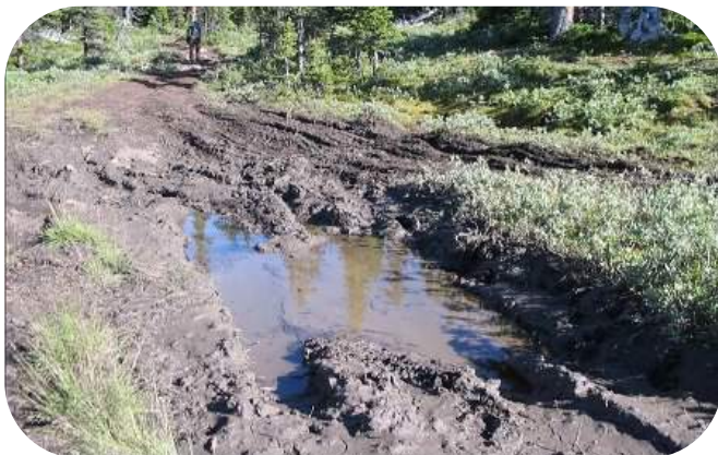
Figure 3: Trail degradation due to a combination of poor water drainage and excessive motorized traffic in the Bighorn Wildland, North Saskatchewan River Basin. From AWA 2007.
